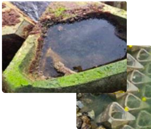
Pilot study of ECONcrete Coastallock armor units in the San Diego port 88
